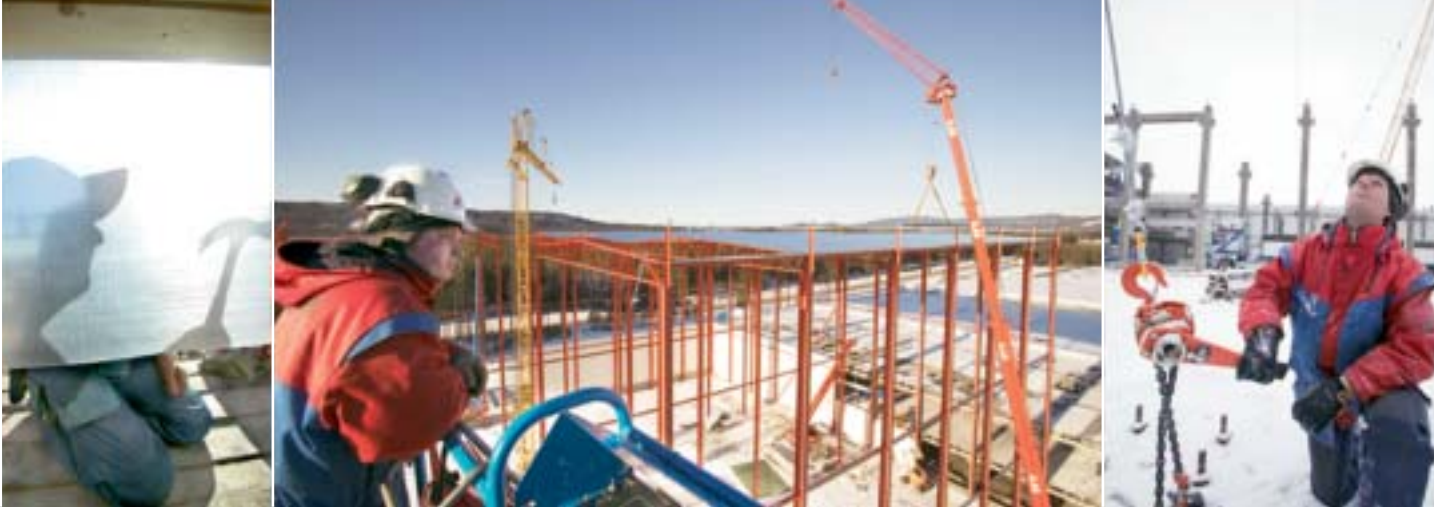
WINTER IN INSJÖN 2004—WORK ON EXTENDING OUR CENTRAL WAREHOUSE IN FULL SWING.
